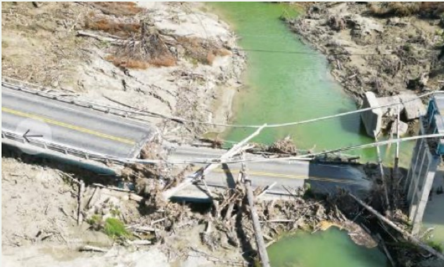
DOWN BUT NOT OUT: Hikuwai Bridge No 1 collapsed in Cyclone Gabrielle in February, taking with it critical fibre connection for the East Coast. A fibre bypass has been completed. Picture by Rory O'Sullivan, Chorus
